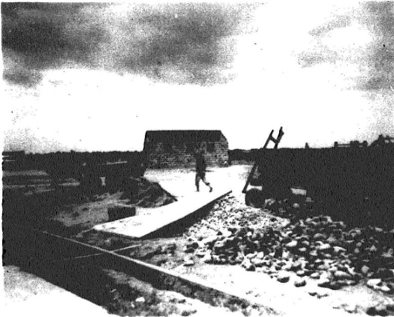
Construction of Latrine, Tao Yuan Air Base. Latrine Under Construction Shown in Background.
